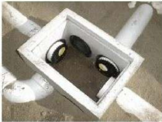
The Inlet Pipe Is On the Right
